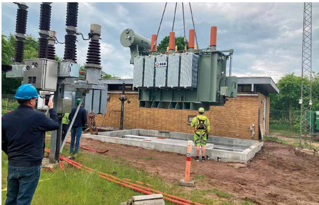
Station Give – udvendig ny transformer
